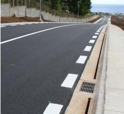
Fig 2. Collecting of road runoff by a slot channel
