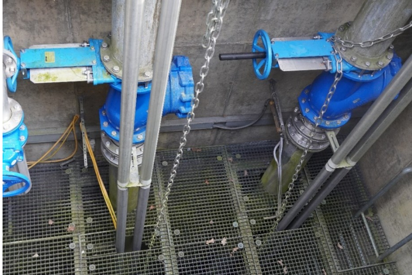
Figure 3: First water collection tank and pumps, which are activated after a certain water volume is reached.
