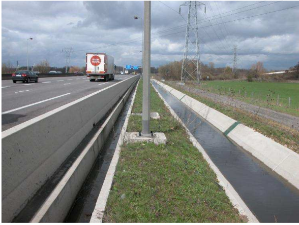
Fig 3. Collecting of road runoff by a U-shaped channel
