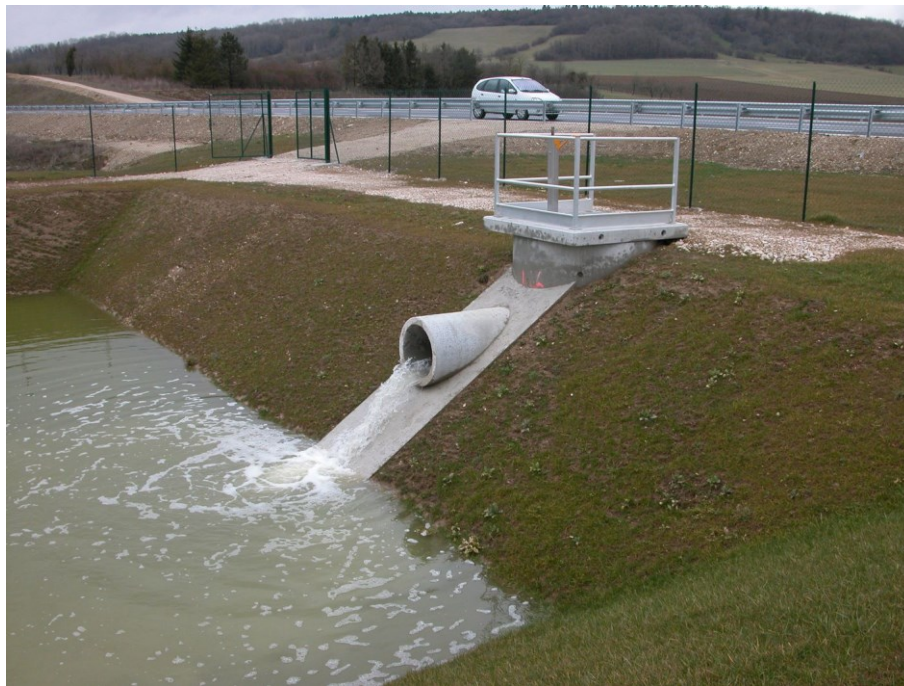
Figure 1: Water arriving in a basin (Cerema)
